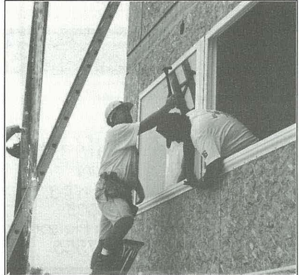
Rod Jones and Ron Johnson install a window in the new press box. Photo by David Campbell.
